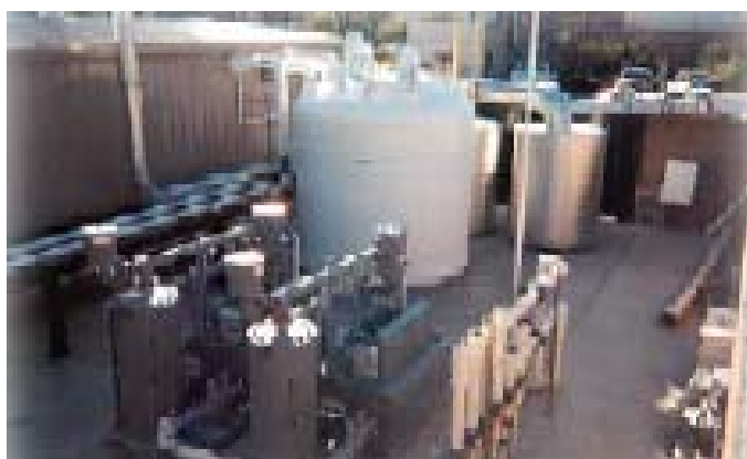
Figure 2. Area 7 Air Stripper/GAC Filter System
